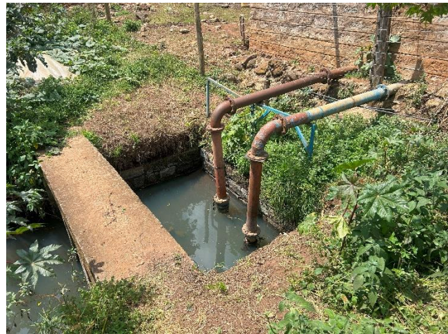
Figure 9: two inlets at Flamingo intake (own photo)
